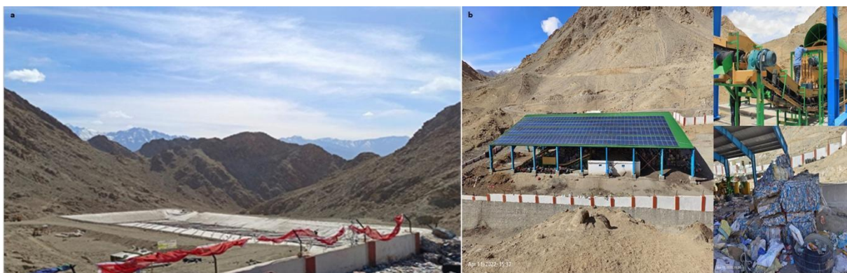
Figure 6. (a) Establishment of solar power-based solid waste management plant: A new initiative by Ladakh (UT), and (b) Landfill area under construction near Solid Waste Management Plant Skampari, Leh
